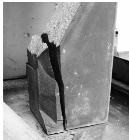
Fig. 6b) Overlay failure detail
