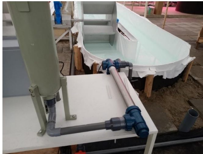
Figure 21 – UV filtration system utilized to eliminate undesirable microorganisms and maintain water quality within cultivation tanks. Photo: Paulo Pereira
