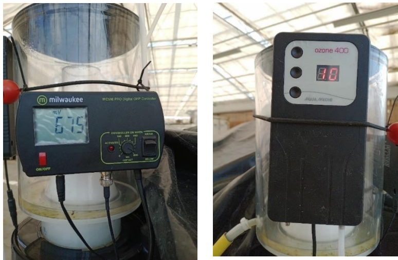
Figure 37 – Monitoring system showing the Milwaukee Digital Controller (left) and the AquaMedic Ozone 400 system (right). Photo: Paulo Pereira.
