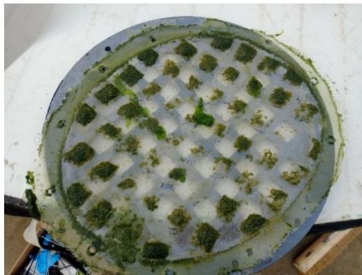
Figure 48 - Blocked drain in Ulva Raceway. Photo: Paulo Pereira.
