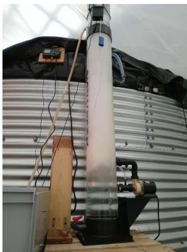
Figure 39 – AquaMedic Turboflotor 5000 skimmer installed in the reservoir tank for particulate matter removal and ozone injection. Photo: Paulo Pereira
