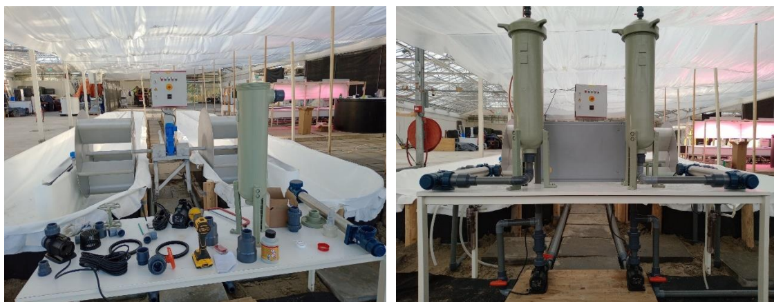
Figure 20 – Construction and completion stages of the filtration system designed specifically for the 10,000 L raceways, featuring mechanical filtration to remove particulate matter and ensure optimal water quality. Photo: Paulo Pereira
