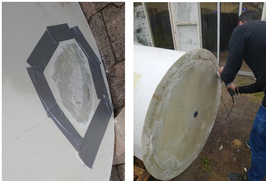
Figure 24 – Maintenance and repair work on fiberglass cultivation tanks, involving resurfacing and sealing to prevent leaks and extend tank durability. Photo: Paulo Pereira
