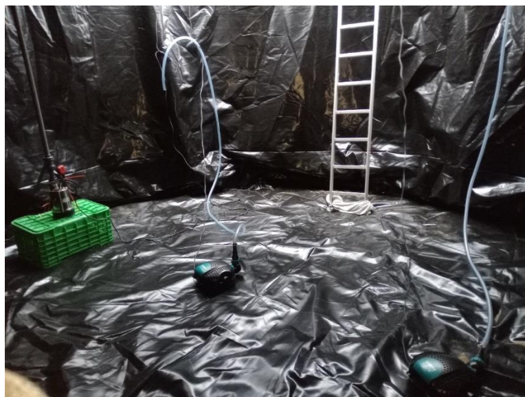
Figure 22 – Recirculation pumps strategically positioned at the opposite end from skimmers, ensuring effective circulation and homogeneous water conditions within the storage reservoir. Photo: Paulo Pereira
