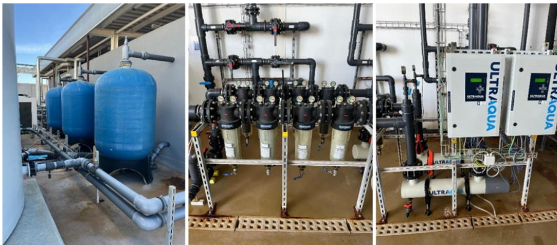
Figure 7. The three-stage filtration, sand filters (left), cartridge filters (middle) and UV filters (right) (Source: Author, 2025).
