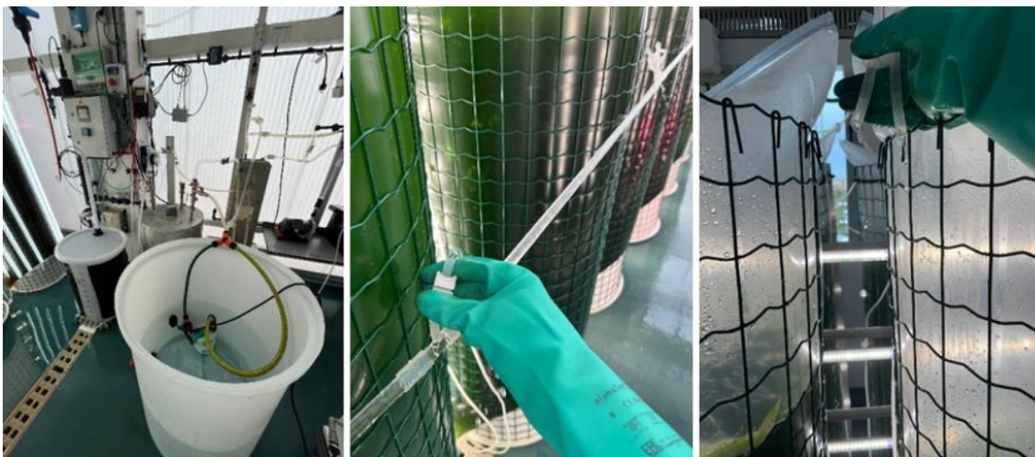
Figure 27. Acid and sodium hypochlorite cleaning: solution tank and cleaning pump (left), loading the lines (middle) and, solution dripping from the capillaries (right) (Source: Author, 2025).
