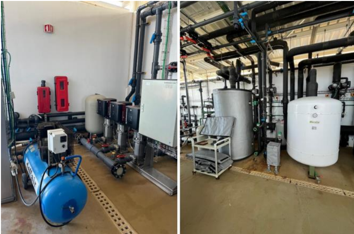
Figure 8. Technical area' water pumps (left) and heaters (right) (Source: Author, 2025).
