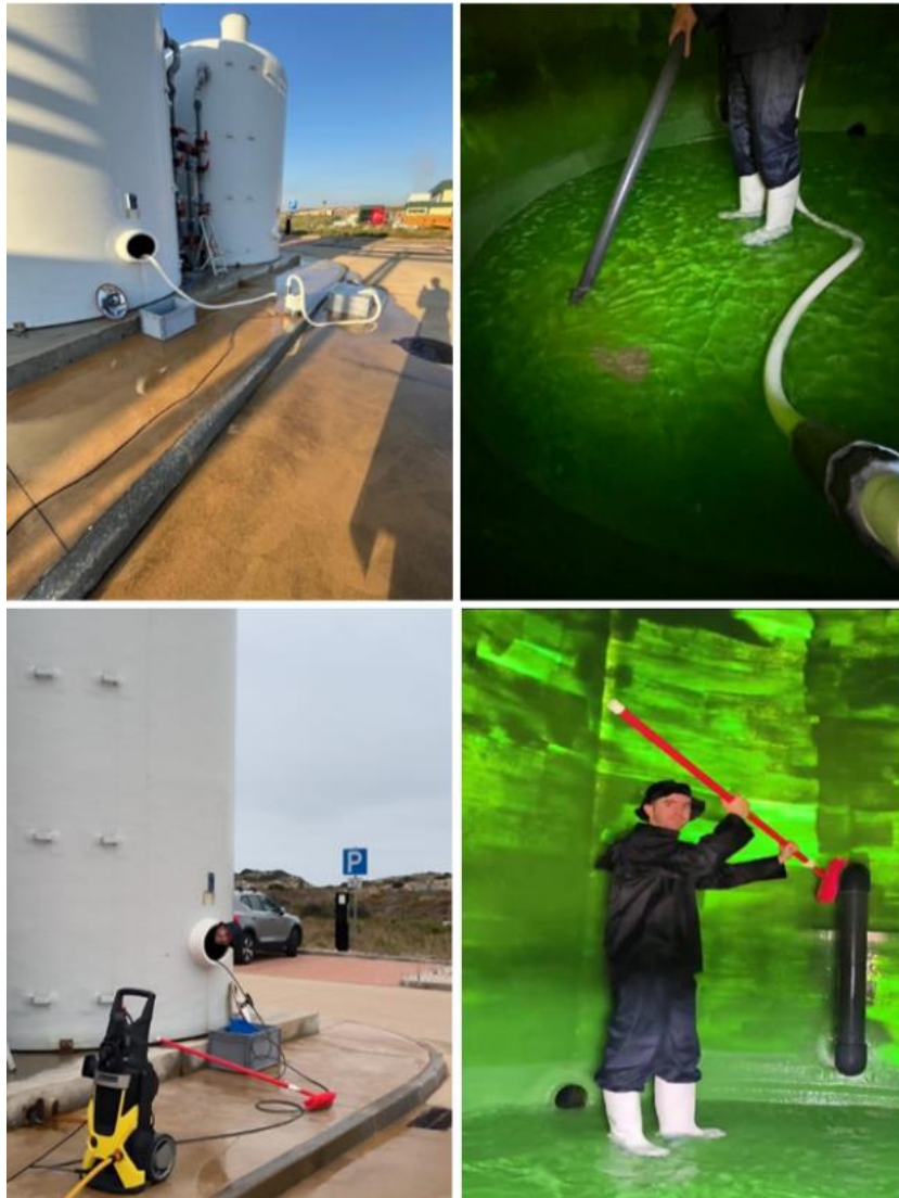
Figure 9. Reservoir cleaning operation – access via opened hatch (top left), deposits suction (top right), cleaning equipment (bottom left) and wall cleaning (bottom right) (Source: Author, 2025).
