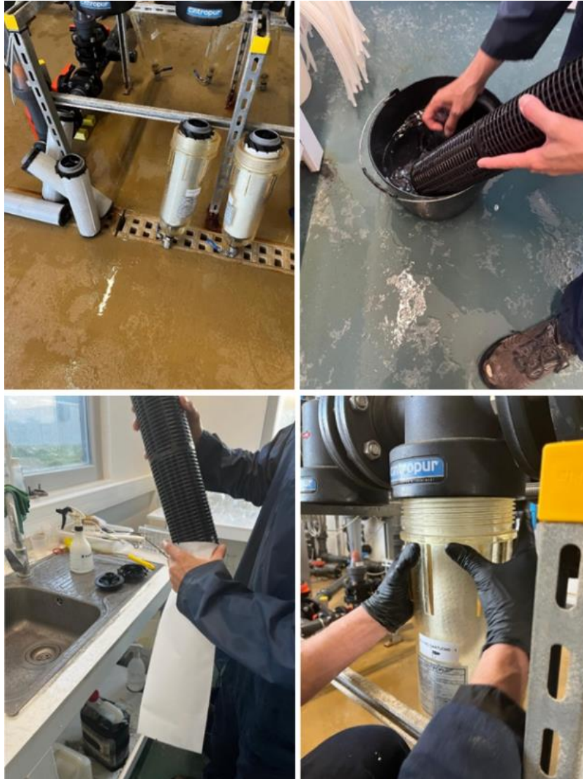
Figure 10. Cartridge filter replacement operation – removing used cartridges (top left), cleaning them with sodium hypochlorite (top right), putting new filter (bottom left) and installing the cartridge in the new line (bottom right) (Source: Author, 2025).
