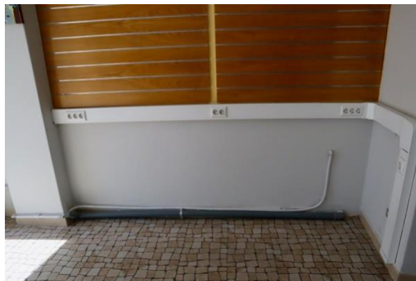
Figure 15 electric scooter charging station
