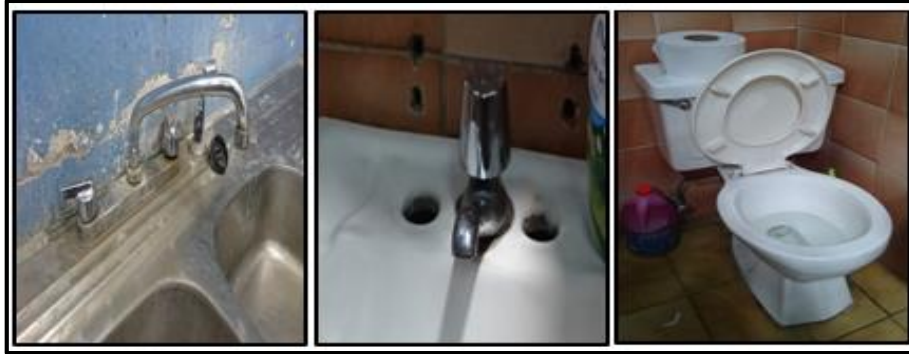
Figure 4.31 - Teacher’s Bathroom – Hydraulics Laboratory
