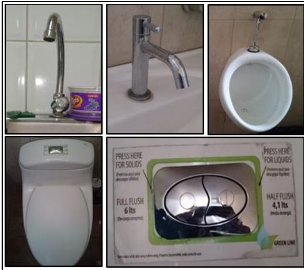
Figure 4.24 - Bathroom's devices (Teacher's bathroom) – Ground Floor
