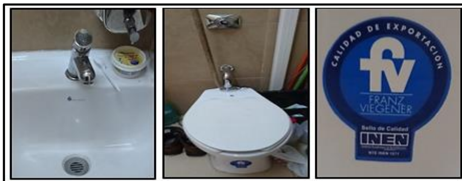
Figure 4.23 - Bathroom's devices (Concierge) – Ground Floor
