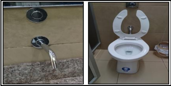
Figure 4.26 - Bathroom's devices (Women) – Second Floor Source: Author's own inspection
