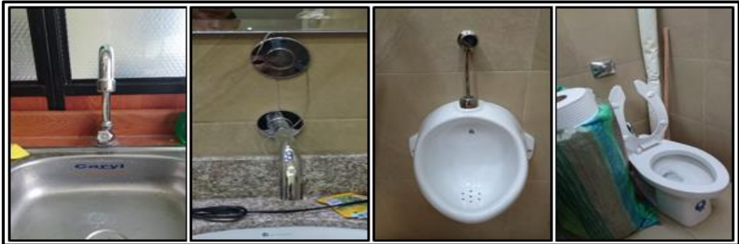
Figure 4.28 - Bathroom's devices (Concierge) – Second Floor Source: Author's own inspection
