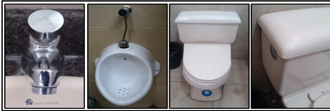
Figure 4.30 - Bathroom's devices (Men) – Third Floor
