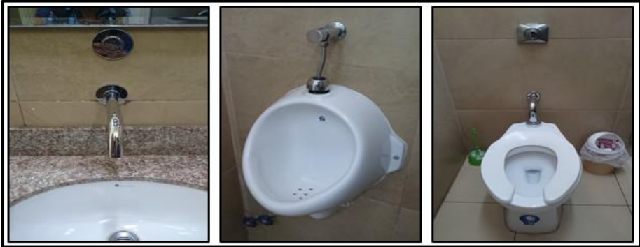
Figure 4.27 - Bathroom's devices (Men) – Second Floor Source: Author's own inspection
