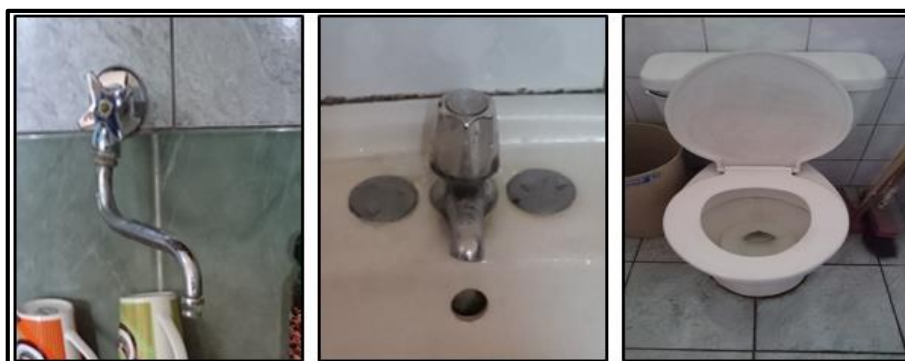
Figure 4.25 - Bathroom's devices (Library Personnel) – First Floor
