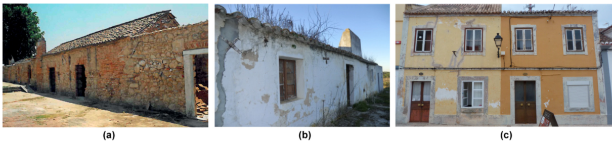
Fig. 12. Ties in Portuguese vernacular architecture: (a) Alcácer do Sal (photo by Mariana Correia, 1997); (b) Melides (photo by CI-ESG, 2013); and (c) Vila Real de Santo António.
