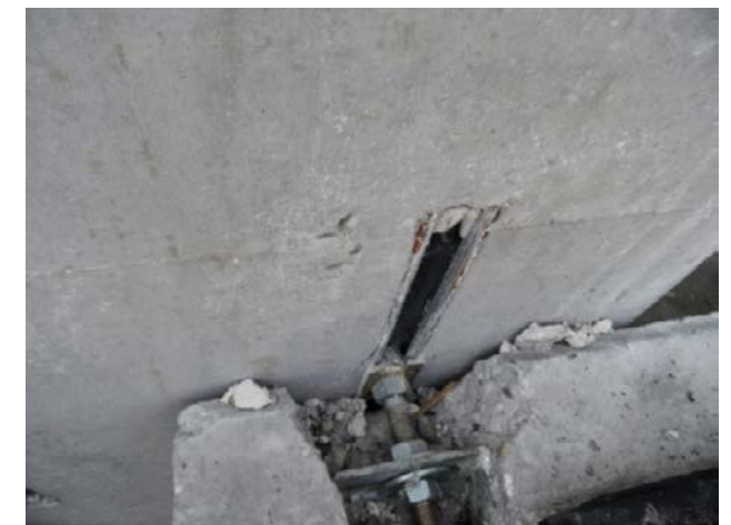
Figure 8 · Top view of the cladding-to-column connection failure [16]
