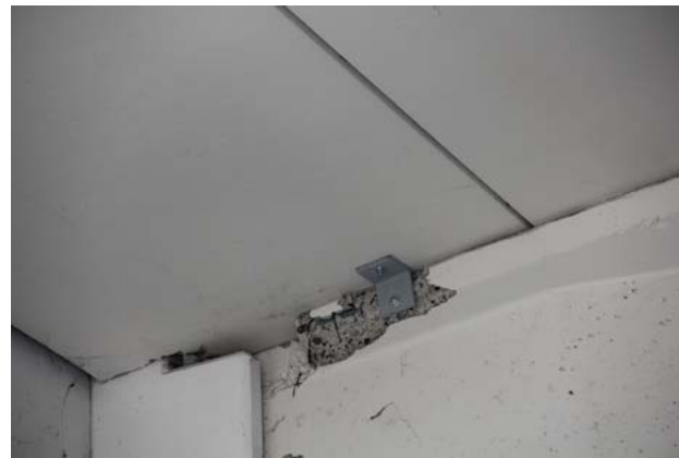
Figure 7 · Beam damage due to the roof-to-beam connection
