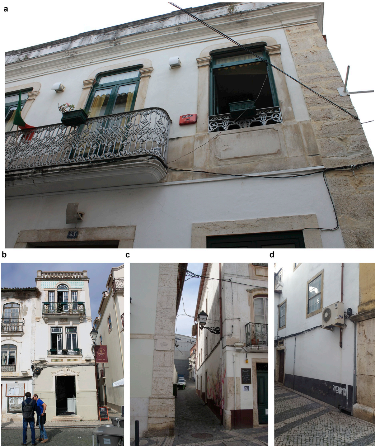
Fig. 3. Non-structural elements connected to the façades: (a) Cornice at the top of a building; (b) typical stone balcony, (c) light elements; (d) air conditioning systems.
