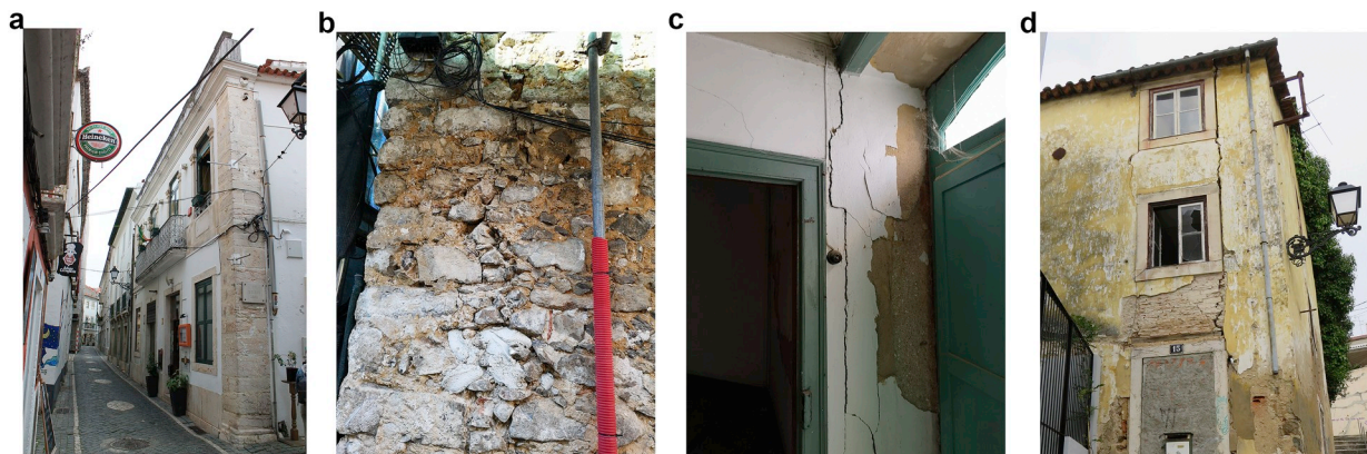
Fig. 5. Connections between structural elements: (a) Good quality connection; (b) bad quality connections between orthogonal walls); (c) detachment crack propagating in the internal corner of the façade; and (d) along the limestone lintels of the openings.
