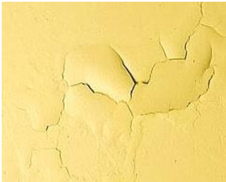
Figure 70: Cracking of paints (Acrylatex Coatings & Recycling, Inc. , 2011)
