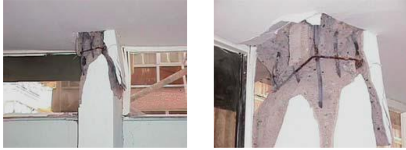
Figure 2.4 – Poor detailing of the reinforcing steel [2].
