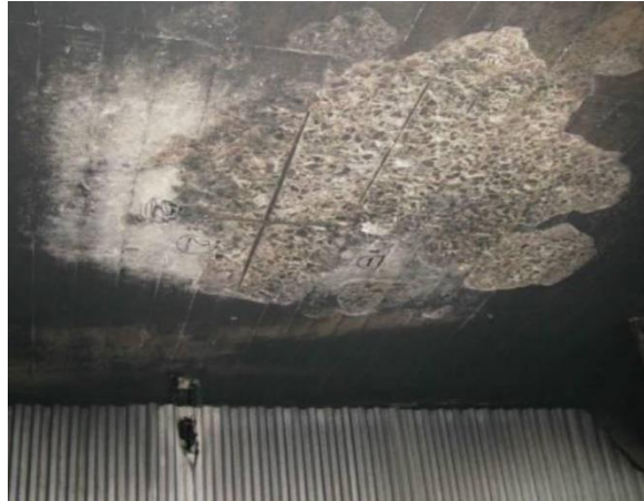
Figure 2.9 – Fire spalling in the roof [12].
