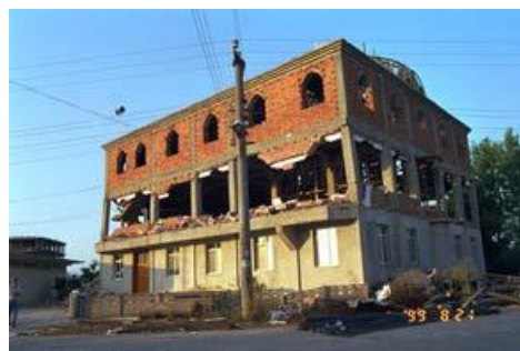
Figure 2.2 – Damage to reinforced concrete buildings with masonry walls [3].
