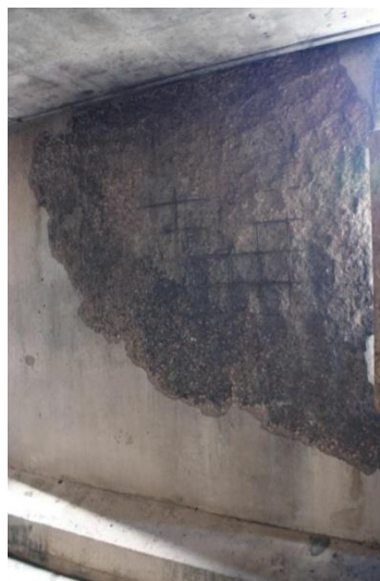
Figure 2.8 – Fire spalling of the external wall [12].
