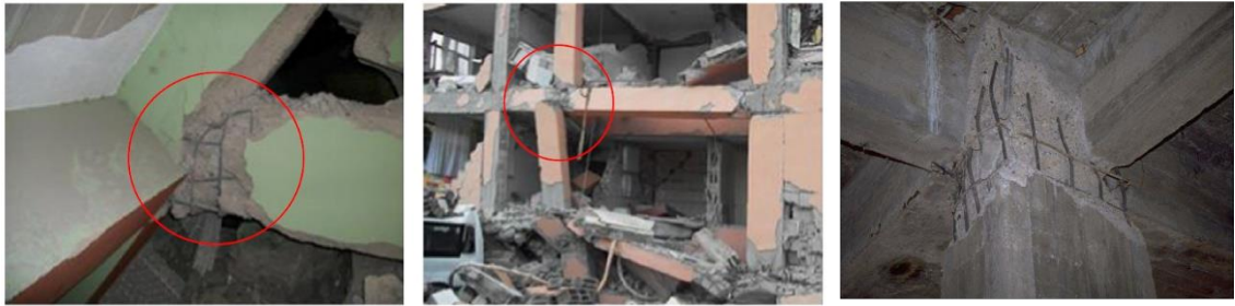
Figure 2.3 – Damage at the beam-column joints. [2][4]
