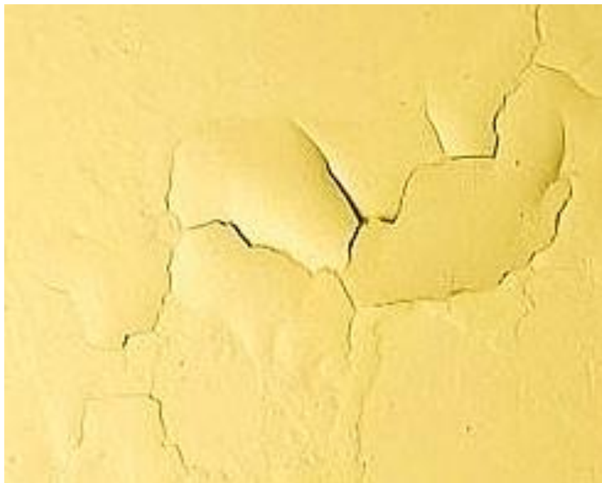
Figure 69: Cracking of paints (Acrylatex Coatings & Recycling, Inc. , 2011)
