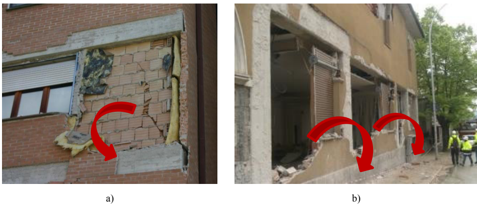
Fig. 1. IM walls earthquake damages in L'Aquila (a) Collapse of the external leaf panel; (b) Collapse of the entire IM wall.
