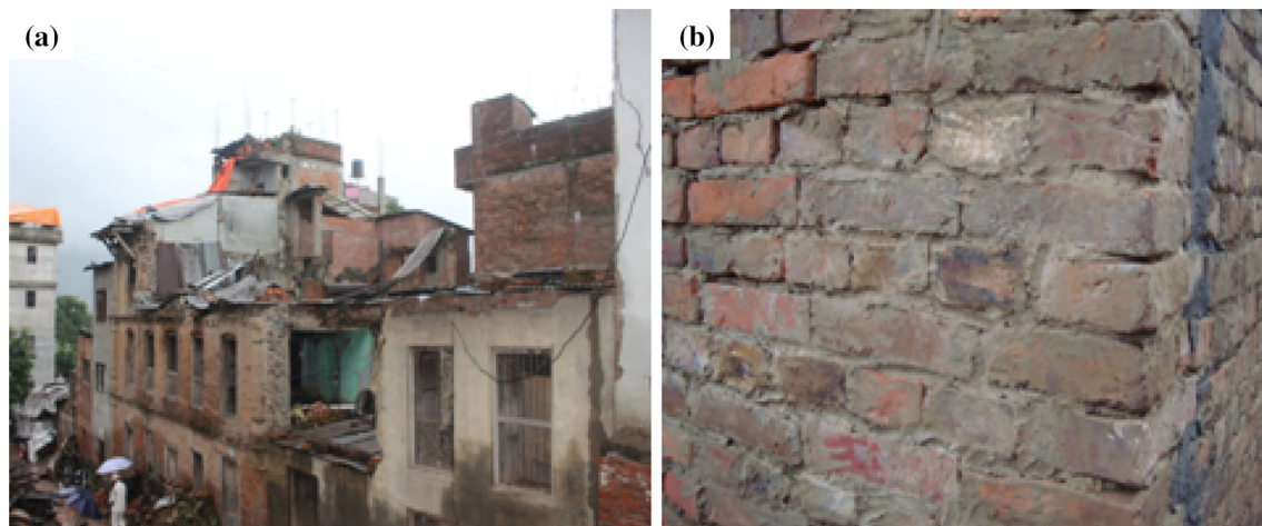
Fig. 11 a Failure of masonry units due to lack of proper binding. b Mud mortar used for reconstruction of URM building destroyed during 2015 Gorkha earthquake at Bhaktapur
