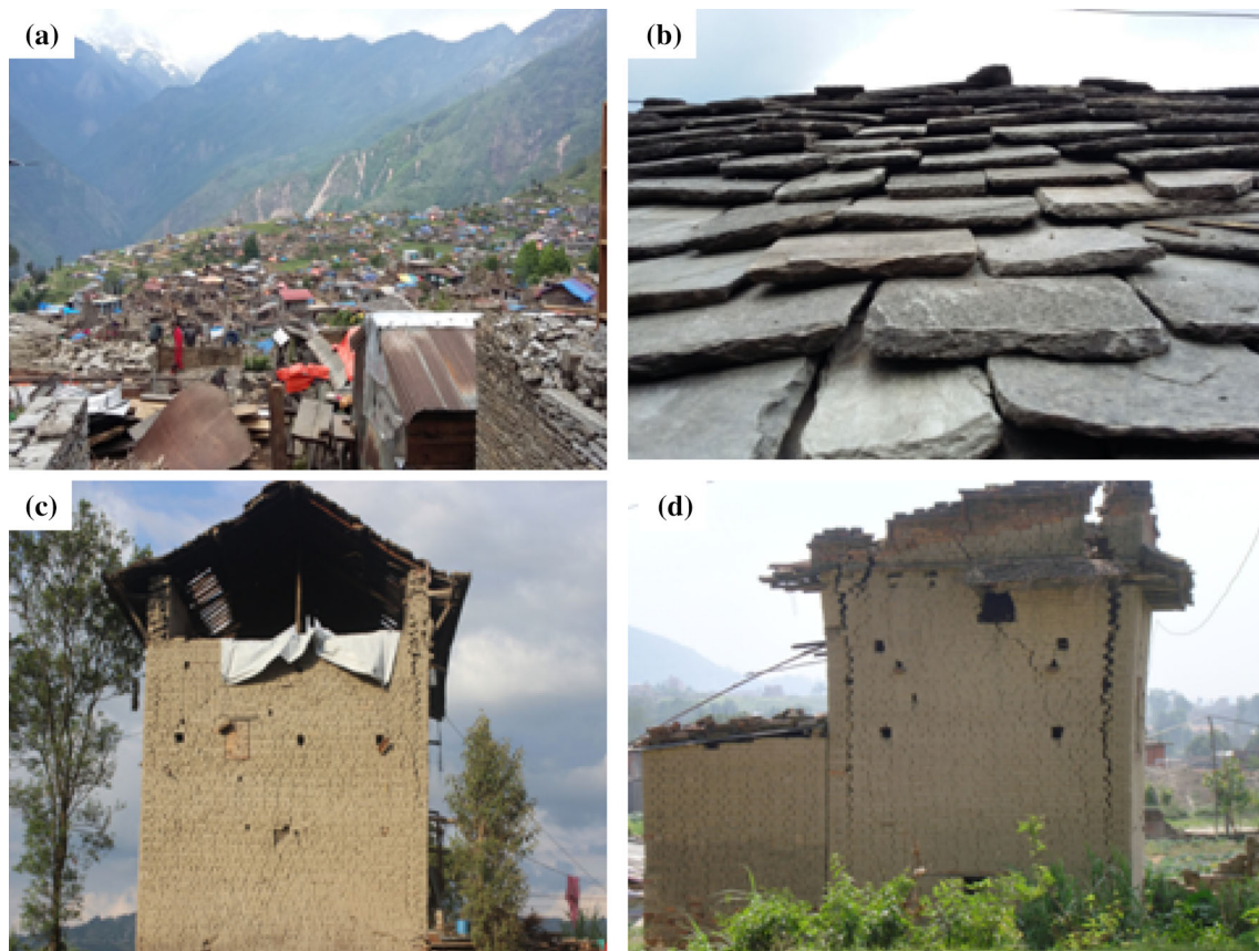
Fig. 16 a Heavily damaged neighborhood of Barpak village where 1250 houses out of 1450 total were collapsed. b Heavy stone roofing in Barpak. c Gable collapse in adobe house in Bhaktapur. d Separation of diagonal walls in an adobe house
