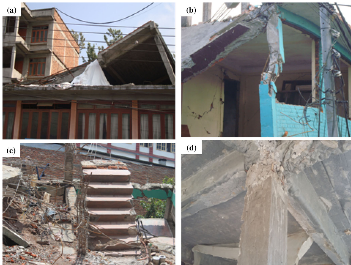
Fig. 2 a Collapsed column due to welded vertical re-bars. b Column failure due to large gap of stirrups. c Outwardly placed 6 mm diameter re-bars exposed on collapsed structures. d Poor beam column connection with exposed re-bars
