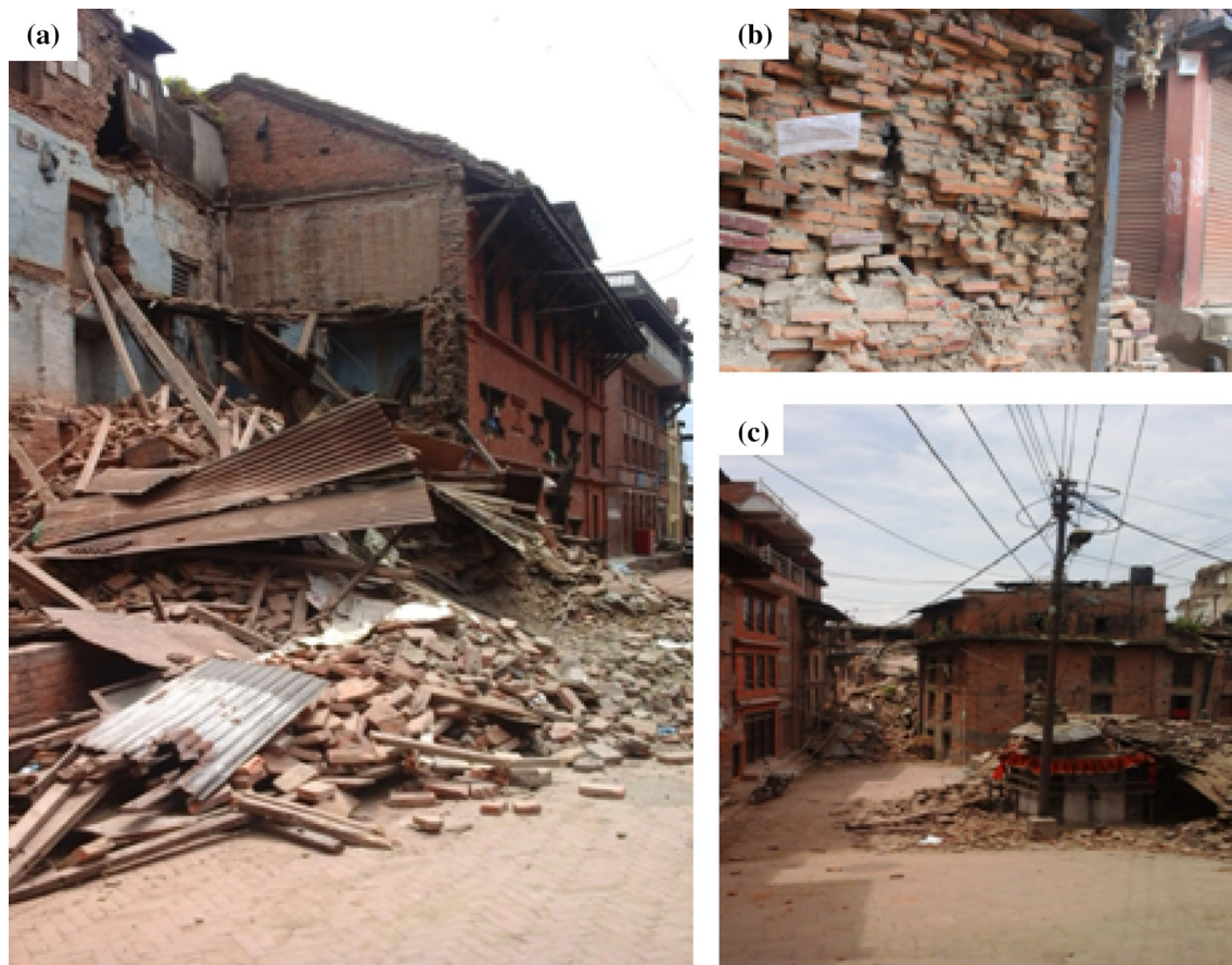
Fig. 13 a Damage in shared wall. b Segregated mud mortar and associated delamination of wythes. c Damaged building with inclined foundation and intact buildings having leveled foundation
