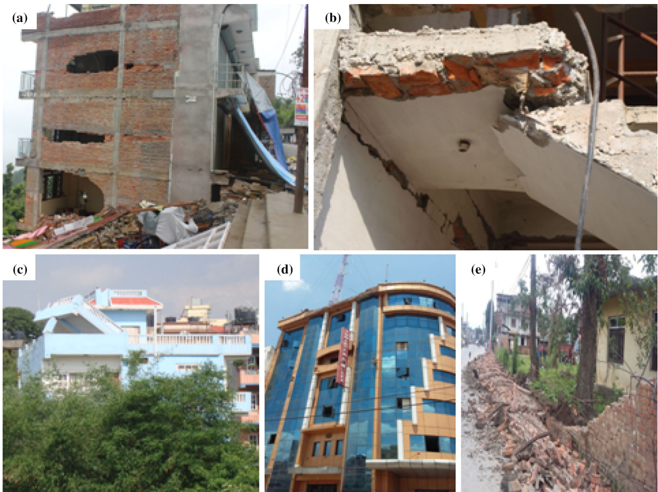
Fig. 8 a Out of plane collapse of brick infill wall in Chautara (Sindhupalchowk). b Damaged staircase. c Damaged water tank. d Damaged parapet wall in a high rise building. e Damaged boundary wall
