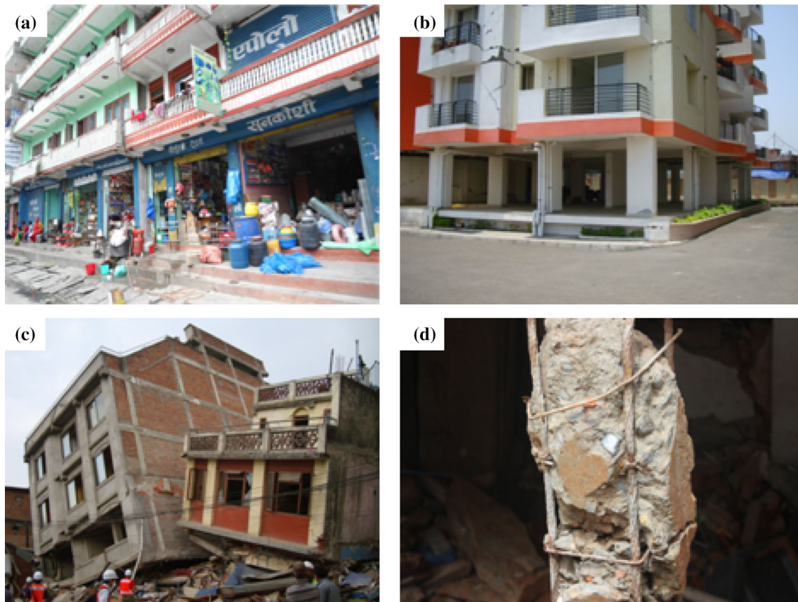
Fig. 1 a Ground floor of residential buildings without infill walls. b Ground floor of an apartment building without infill wall. c Soft storey and structural pounding failure. d 16 mm diameter rebar but only four in number (corroded as well) from a collapsed building in Kathmandu
