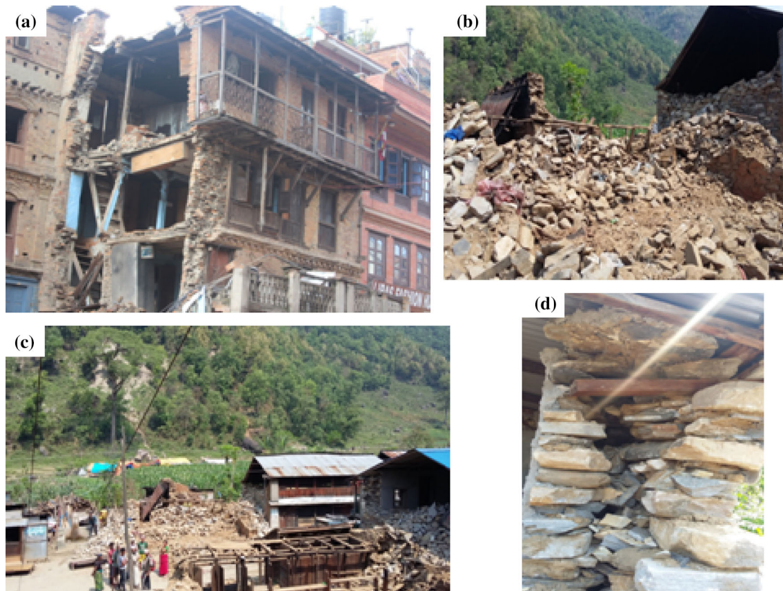
Fig. 15 a Pounding and progressive failure on the building situated on edge. b Complete collapse of row houses in Baluwa (near epicenter). c Progressive failure on row houses and good performance of timber frames. d Separated wall due to structural pounding
