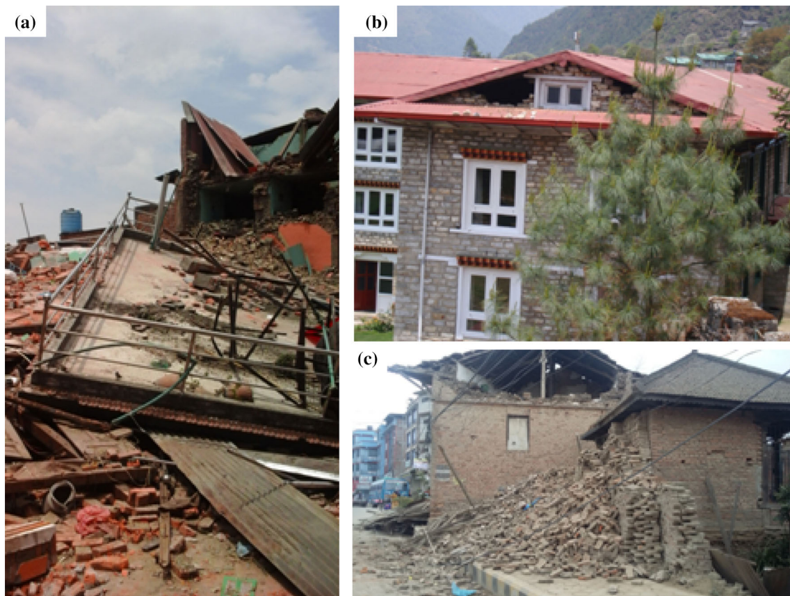
Fig. 14 a Complete collapse of RC slab used as roofing in a masonry building. b Out of plane failure of gable portion of a stone masonry building. c Heavy gable portion out of plane failure in brick masonry
