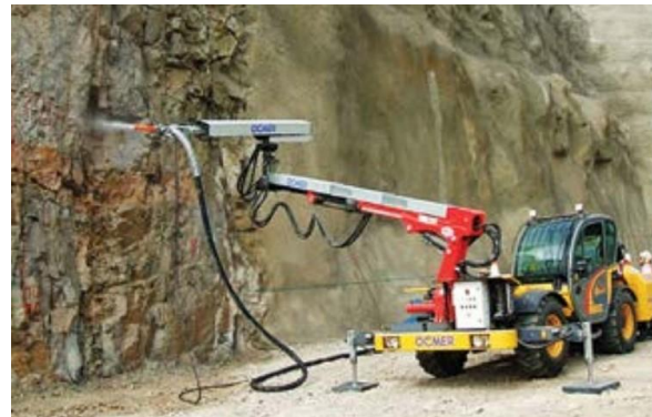
Figure 2.2: Shotcrete where the control of the nozzle pose is done by an operator (taken from [24]).
