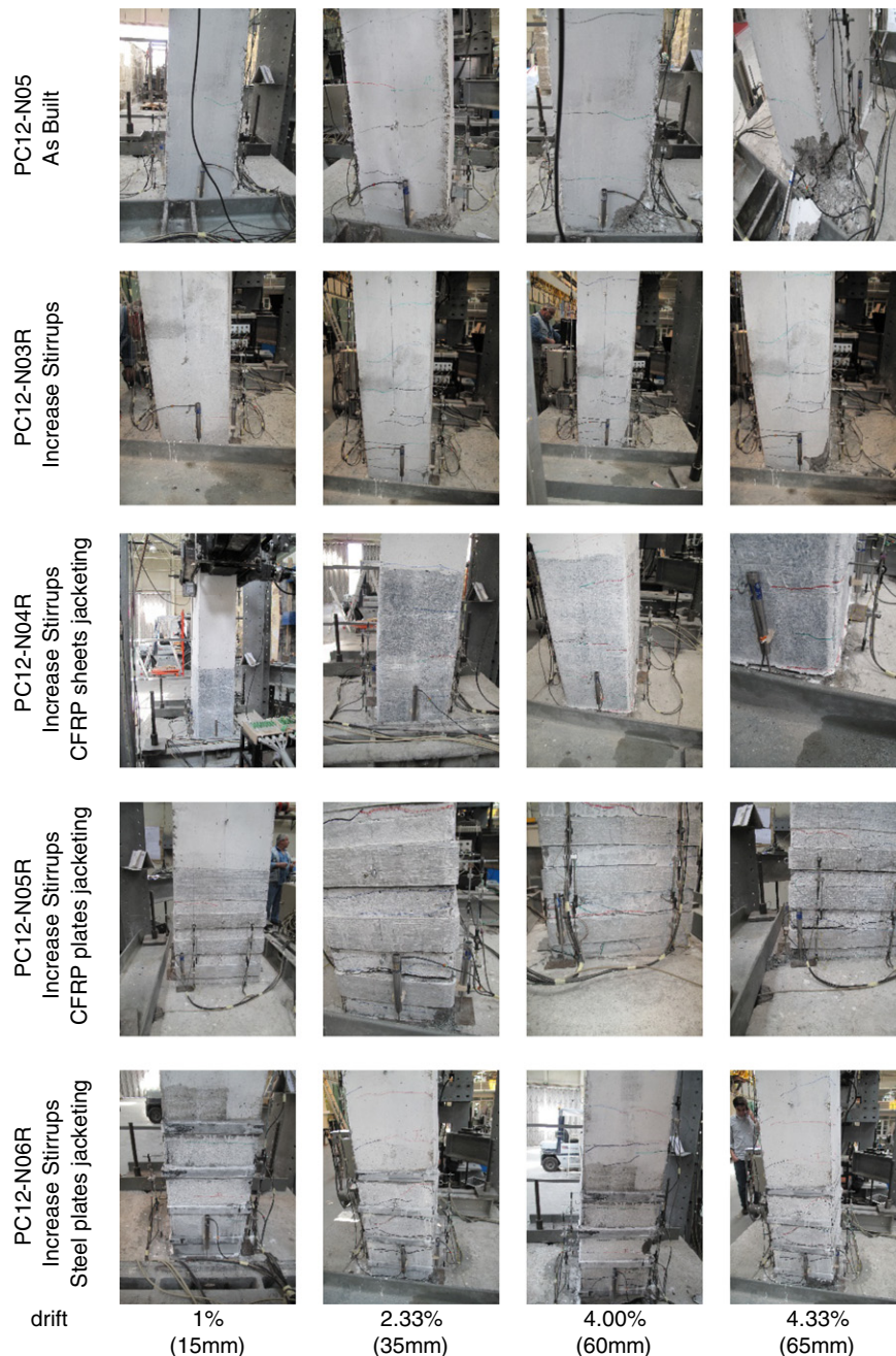
Fig. 15. Damage evolution in the columns of the all retrofitted RC columns (PC12_N03R to PC12_N06R) and the original column (PC12_N05).
