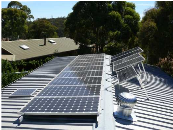
Figure 11: Solar panel lot (Photo: peakpx, CC0 1.0)
