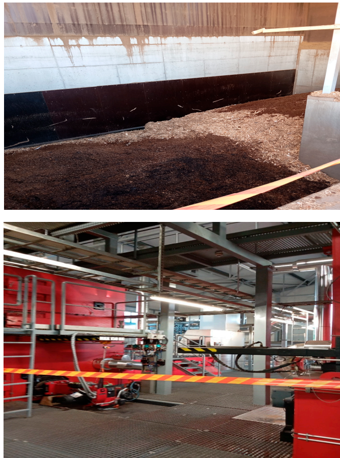
Figure 1. The wood residues container ( top ) and the interior of the plant with one of the boilers ( bottom ).
