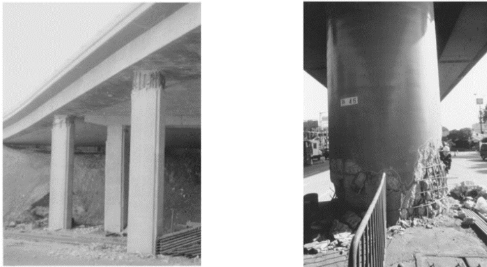
a) San Fernando Road Overhead damage in the 1971 San Fernando earthquake
