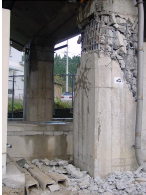
Figure 1.11: Shear failure of a column of Shinkansen bridge. 2004, Japan [40]
